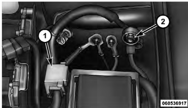
Remote Battery Posts
