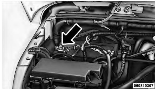
Positive Battery Post
