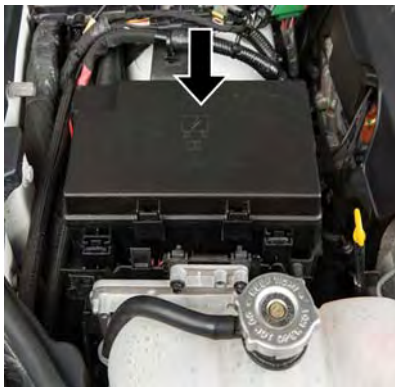
Power Distribution Center Power Distribution Center
