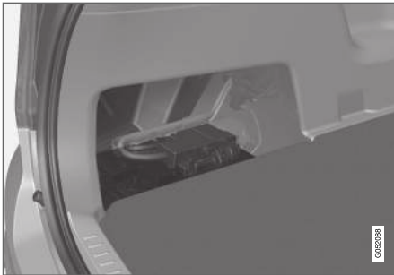
The start battery is located in the cargo compartment.
