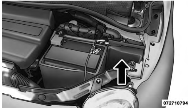
Front Distribution Unit
