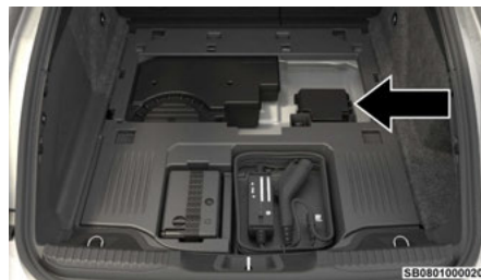
Rear Power Distribution Center
