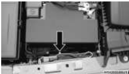
Auxiliary Switch Connections – Under Hood
