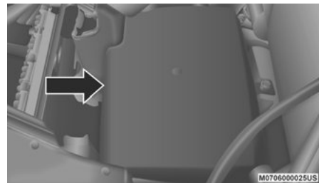
Front Power Distribution Center
